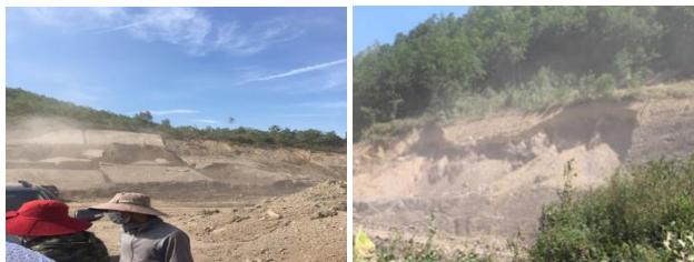
Figure 1. Landslide phenomenon on Route 14G
